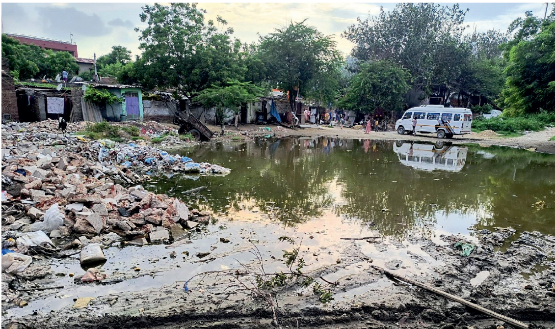
Image 3: Water Logging at Site
